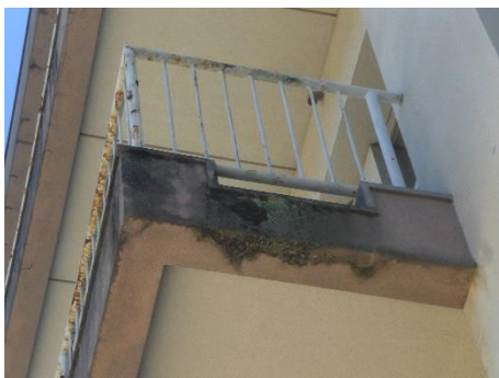
D 判定：錆・腐朽
